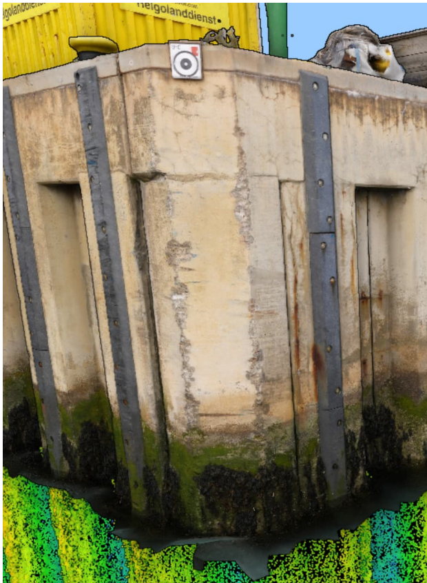
Figure 9. Obvious damages at a quay wall.
