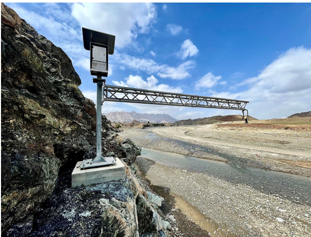
Figure 1. Radar gauging station in Lihban - during low flow conditions
