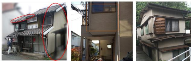
Figure 1. Earthquake-induced building damage
