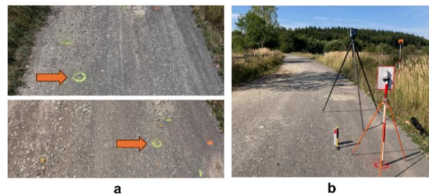
Figure 3. (a) Metal bollards driven into the road surface to serve as GCPs; (b) TLS scanning with checkboard reference targets, which are also installed on the metal bollards.
