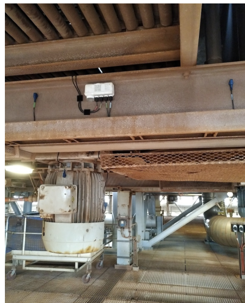
Figure 2. An IoT device and sensor probes deployed in the field
