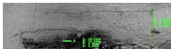
Figure 15. Crack A taken from TLS data in Magnet Collage
