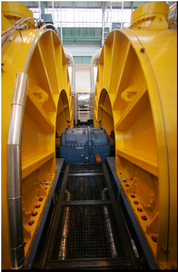
Figure 1. A view of the bearing between the low pressure parts of the turbine with orange bracket for HYNI measuring sensor.
