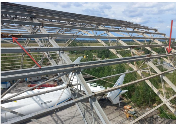
Figure 15. Coverage bar failure.
