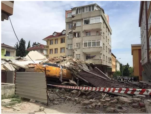
Figure 7. The collapsed building (Web-3)
