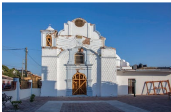
Figure 3. Typical damage of facade and bell towers – Historical Churches September 2017 Puebla, Mexico earthquake
