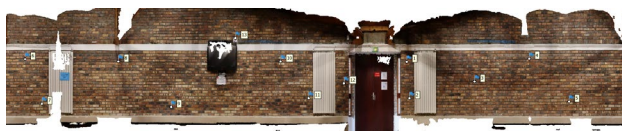
Figure 12. GCP locations (blue flags) on an unfolded image of the rounded tower (inside).
