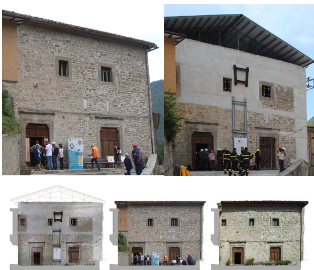
Figure 2 The church façade before (top right) and after (top left) the safety works. Bottom: comparison among the orthophotos: May 2019 (left); August 2016 (centre); before the earthquake.
