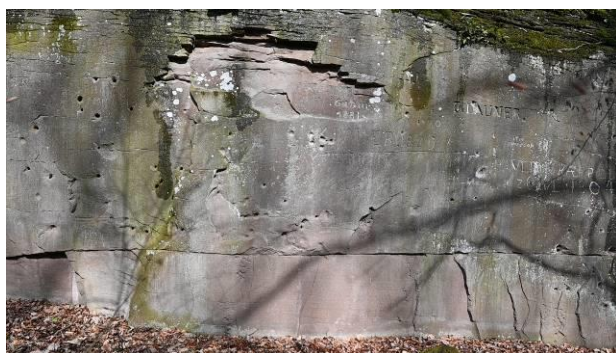
Figure 4. Stone wall with graffiti, bullet holes and a big spalled of part.
