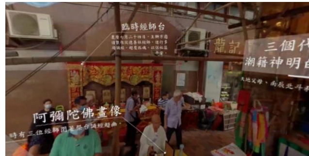
Figure 7. Left hand side of the temporary bamboo scaffolding structure which encompasses the altar
