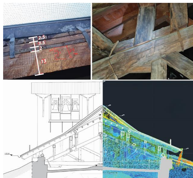
Figure 10. Direct measurements and photographs were additional material necessary to accompany the point cloud for producing technical drawings of the oldest wooden truss roof.
