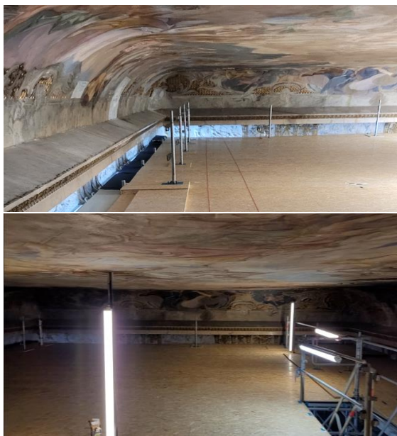
Figure 2. The Festsaal ceiling in the Ansbach Residence, with the scaffolding platform in place.
