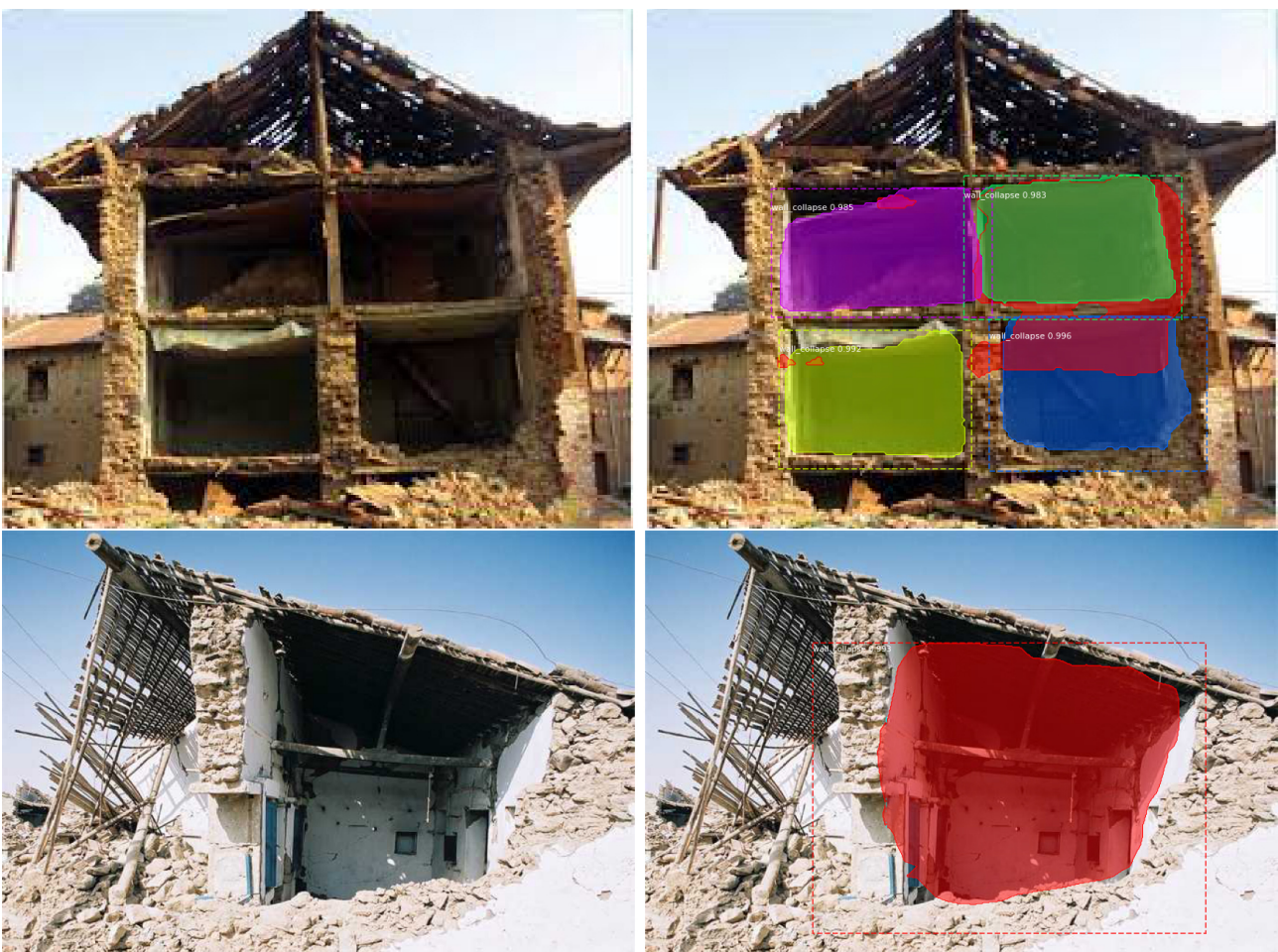
Figure 8. Photos showing the wall collapse damage detection results on random photos of damaged buildings taken from the internet.
