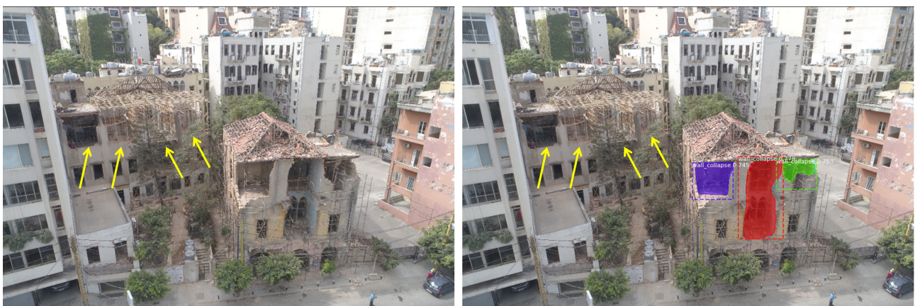
Figure 6. Photos showing the misdetection of some of the wall collapse damage in areas partially covered by trees or by wooden and metallic scaffolding on the inside.
