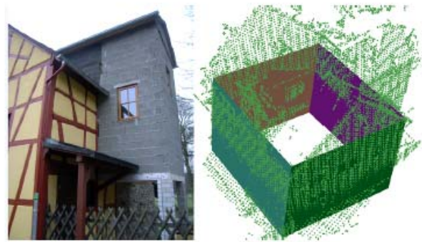
Figure 11: Left: Image of building consisting of four major walls showing balconies or oriels. Right: The derived point cloud consists of 1.6 million points, the four major walls were successfully detected, segmented and connected.
